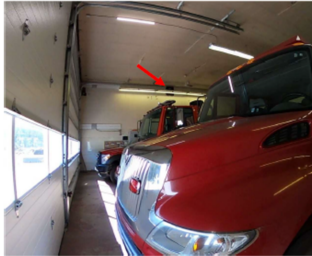
Figure 2: Truck Bay Existing Exhaust Fan
