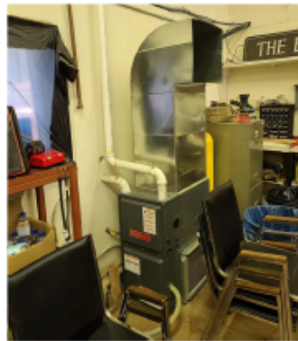
Figure 1: Truck Bay Propane Furnace
